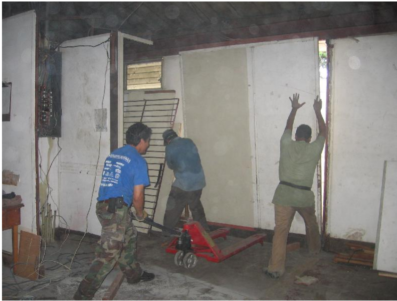
Moises Guillen (in the blue), coordinating the renovation project. Covering the existing warehouse side door.
